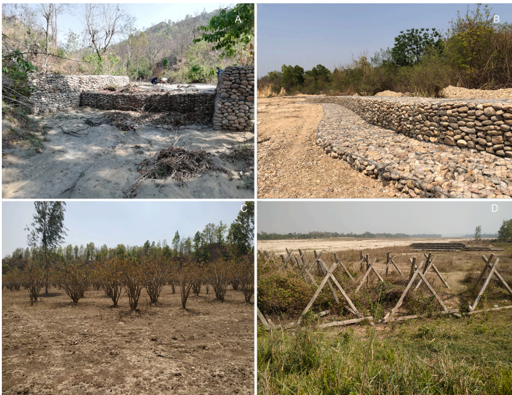
Fig. 2. Representative restoration sites of the Jalad River Basin. A: check dam in river gullies (site 2), B: river embankment (site 12), C: afforestation (site 10), and D: erosion breaker (site 13).
